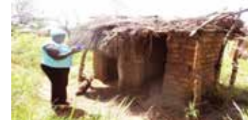
Delapidated sanitation in schools and communities
