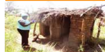
Delapidated sanitation in schools and communities
